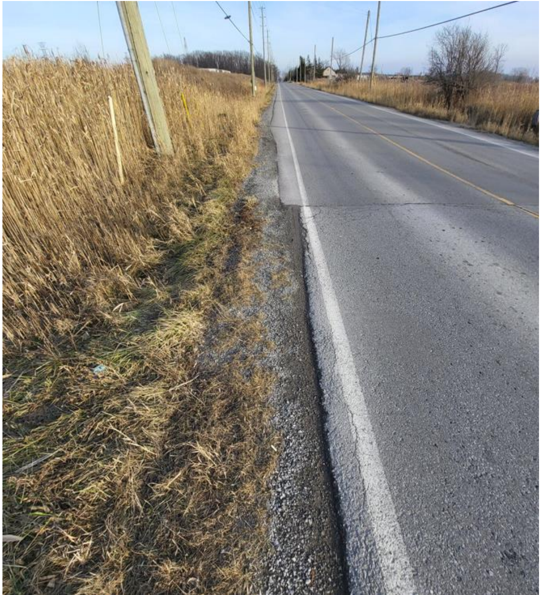
Figure D-4: Barron Road (East) – Shoulder Condition
