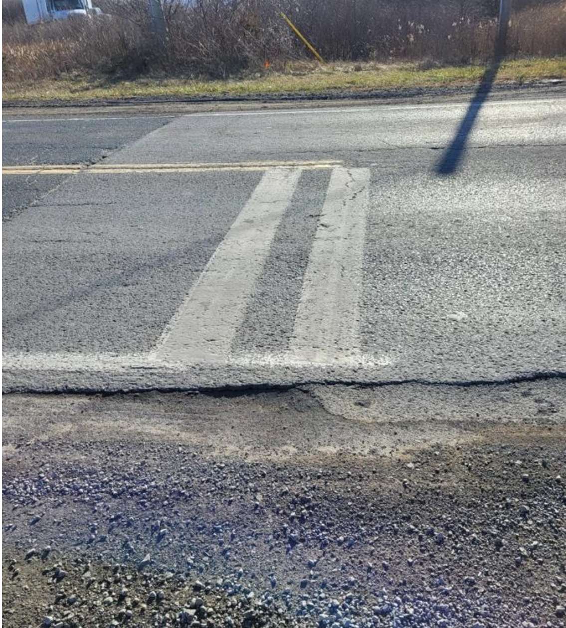
Figure A-14: Lundy's Lane Crossing Stop Bar – Westbound Approach
