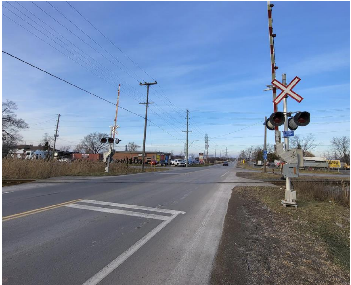
Figure E-2: Allanport Road Crossing – Grade Crossing Warning System
