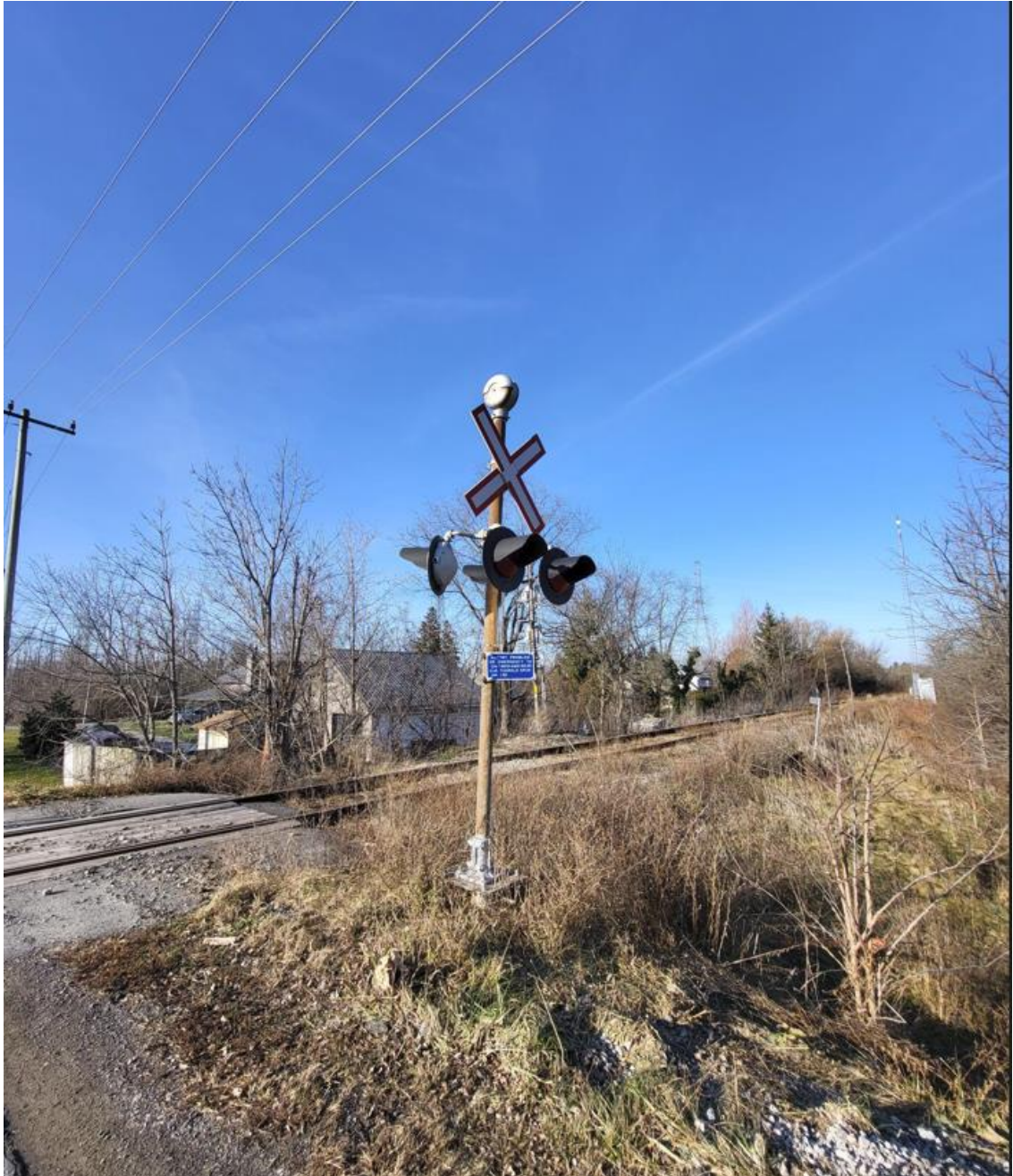
Figure C-16: Barron Road (West) Crossing – Grade Crossing Warning System
