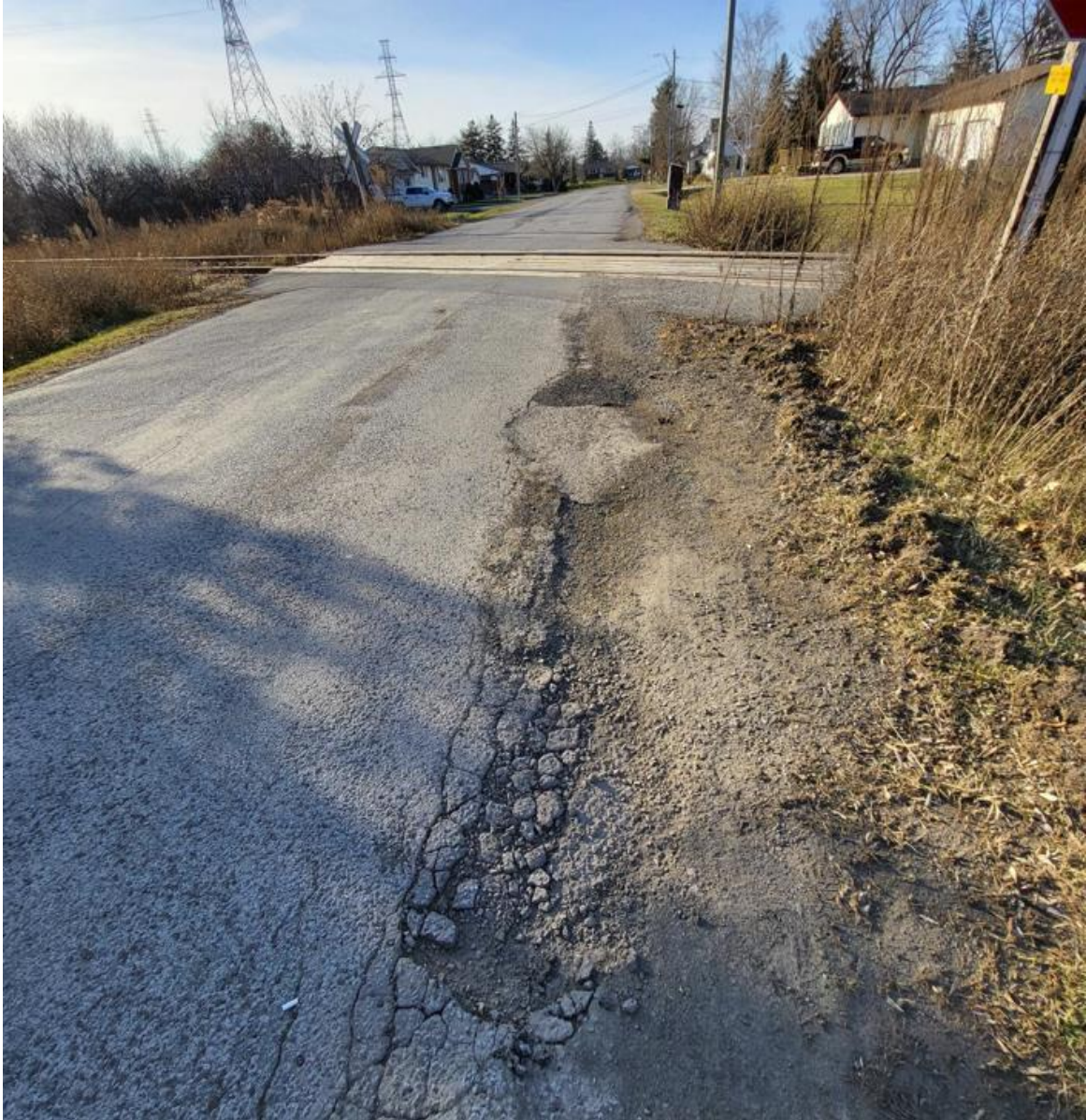
Figure B-2: Henderson Street Crossing – Shoulder Condition
