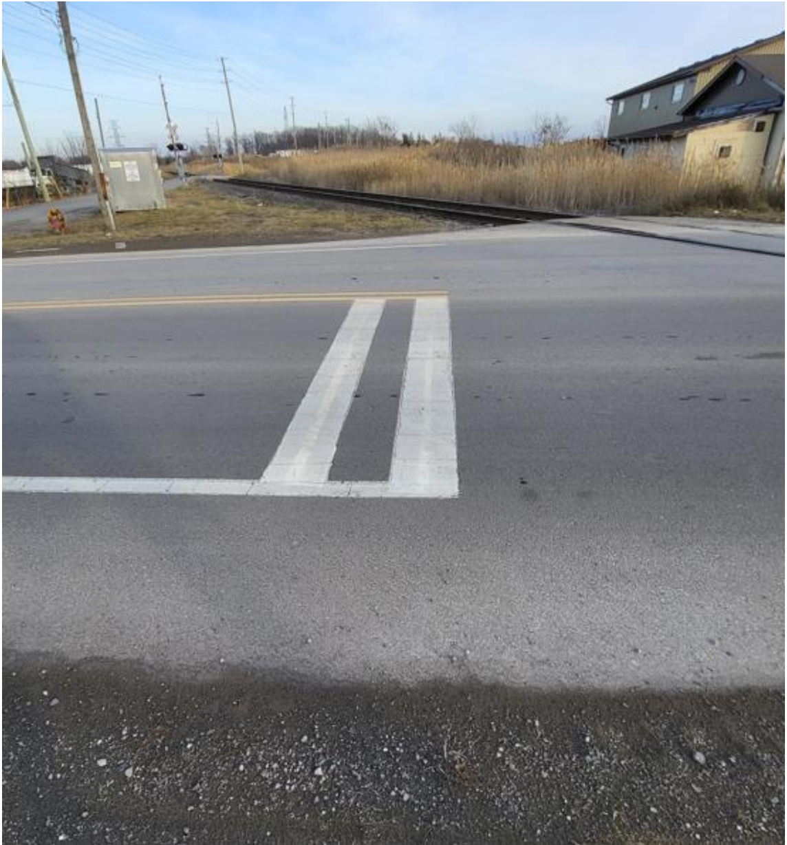
Figure E-13: Allanport Road Crossing Stop Bar – Southbound Approach
