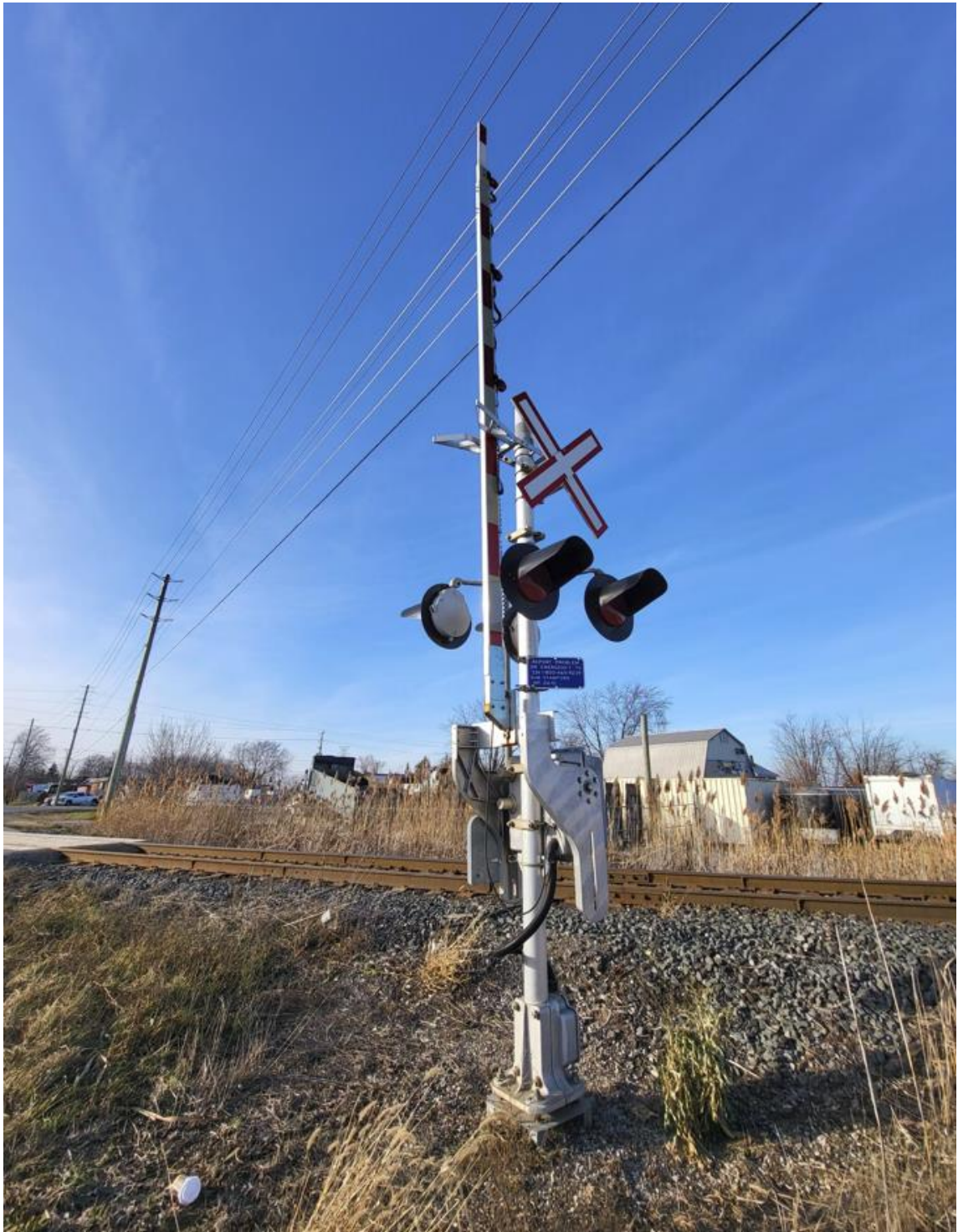
Figure D-12: Barron Road (East) – Grade Crossing Warning System
