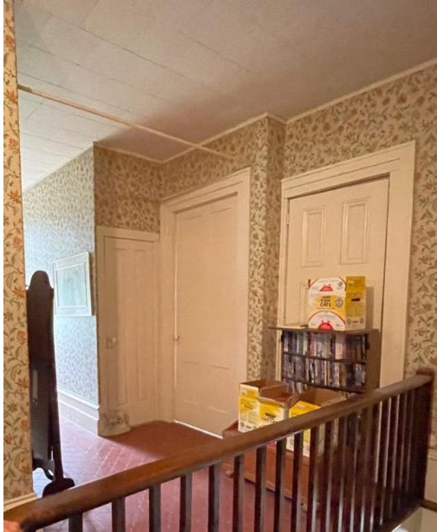
Doors to main façade bedrooms with small closet and showing one of the supporting iron rods
