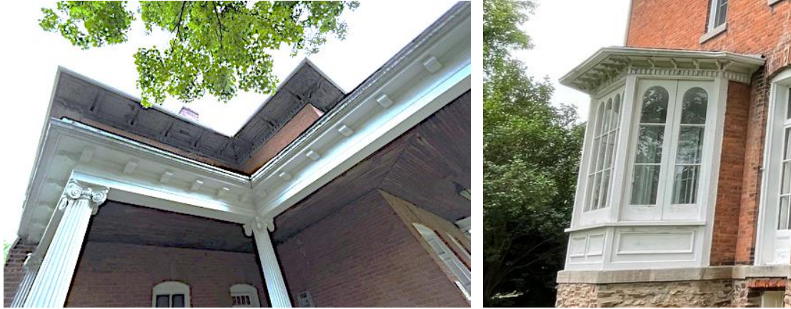
Details of main roof and verandah roof at northwest corner; and above bay window
